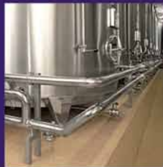
Stainless steel piping
